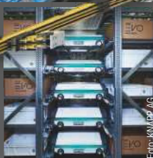
Conductor Rails for Shuttle Systems
